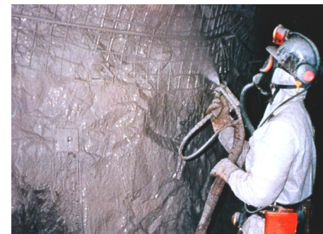
Spray-on plastics liners have been developed by the Department to strengthen rock in underground tunnels.
